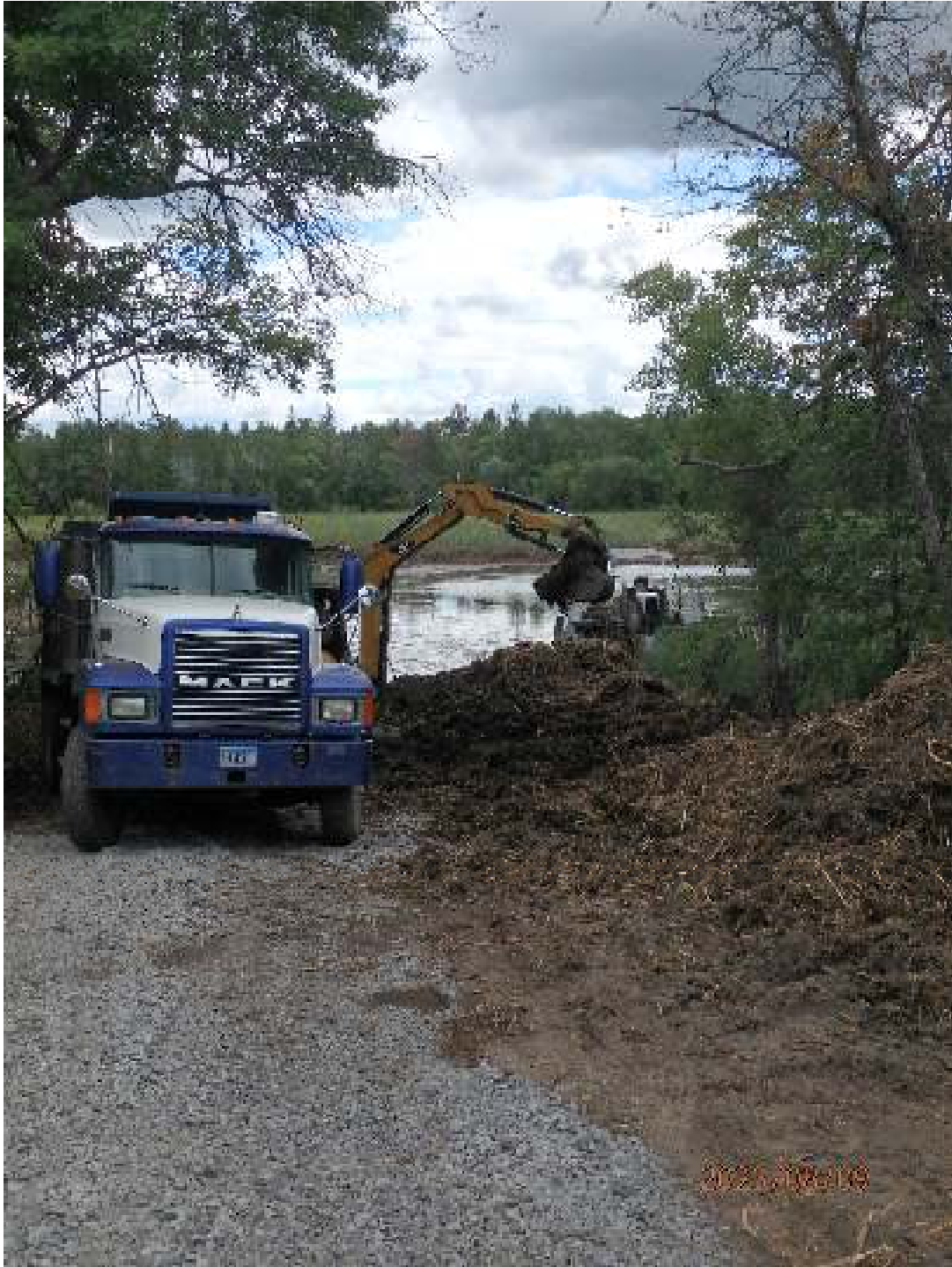
Figure 7 Public access and main staging site for removal and piling of biomass
