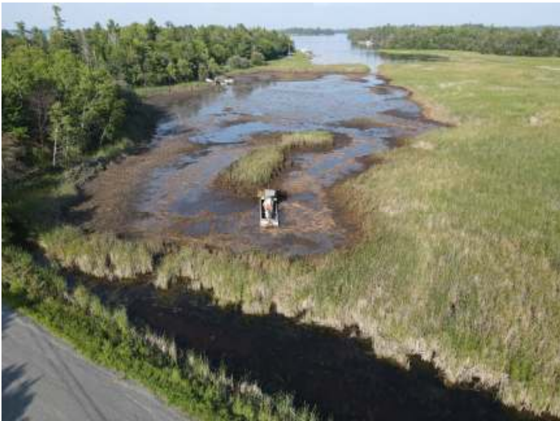
Figure 4 Aerial shot of removal process on the east side of CR134. Photo taken 8/9/2023 by Tom Dougherty
