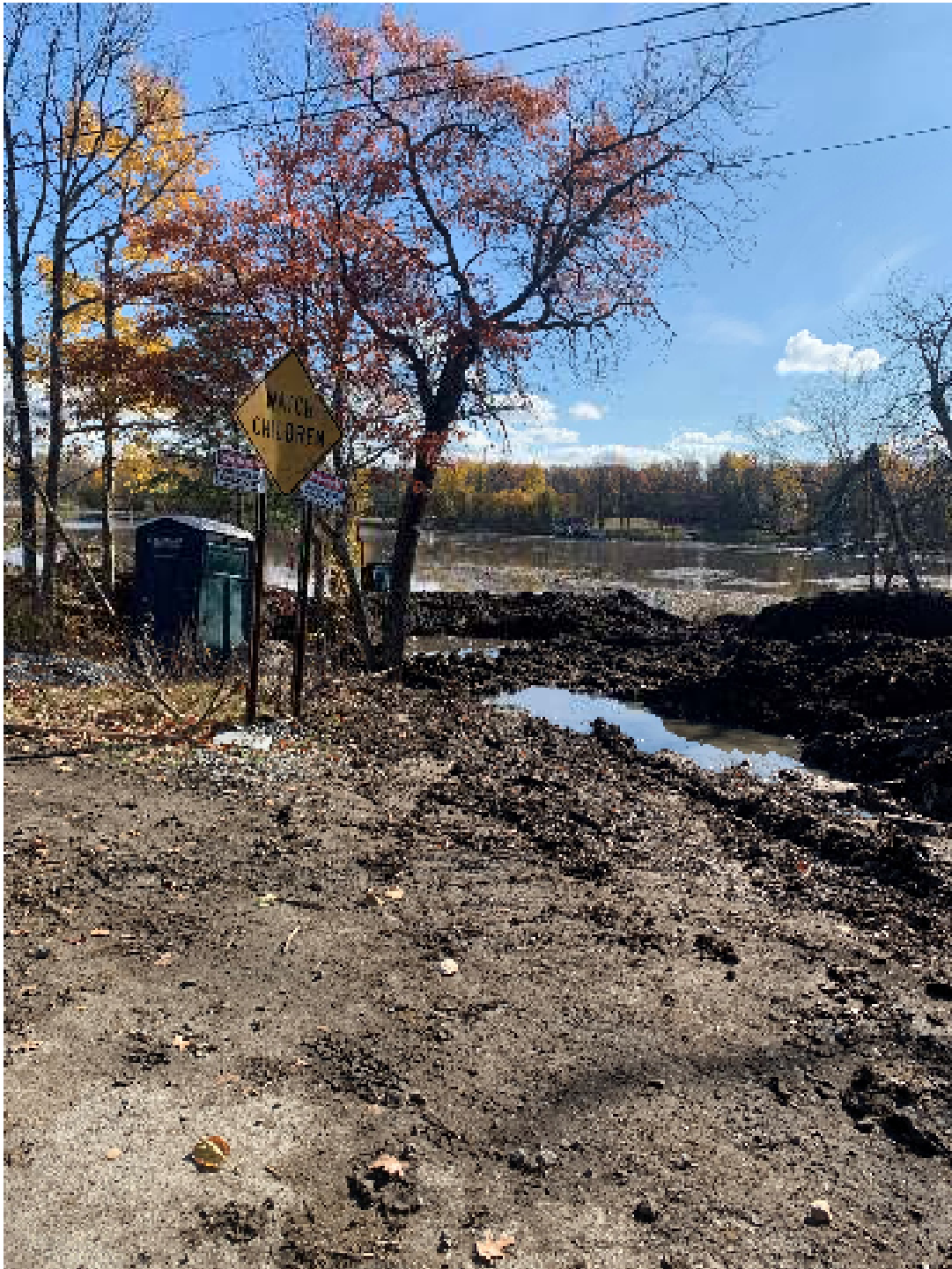
Figure 12 Public access and main staging site for removal and piling of biomass. Photo taken 10/19/2023
