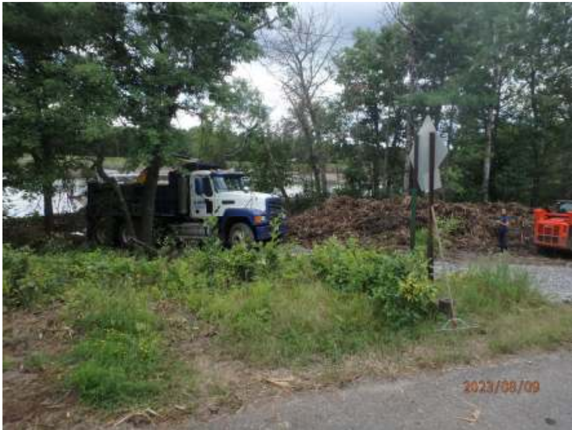
Figure 6 Public access on northeast side of the bay. This access served as the main staging site for removal and piling of biomass
