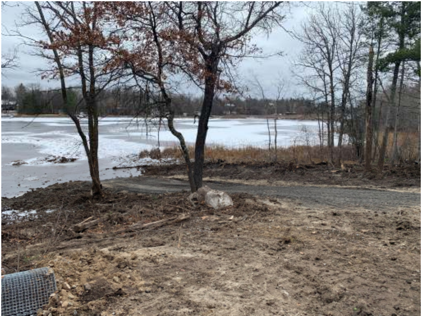
Figure 24 Resurfaced public access. Photo taken 11/2/2023 facing southwest across public access and east restoration area.
